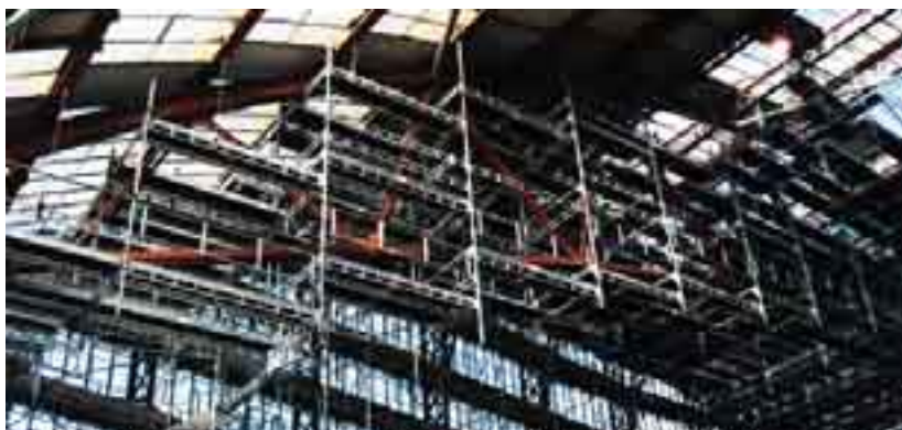
Using suspended scaffolding work can be done on the roof without blocking the floor beneath.
