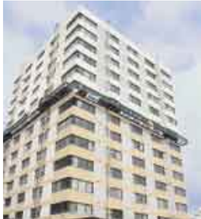
Using a HAKI working platform you will always be at the right place at the right time.
